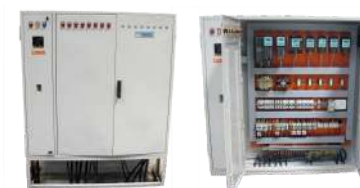
PANEL BOARD FOR EXTRUDER ATTACHED WITH A/C DRIVES FOR WIRE FEEDER & CONVEYOR
